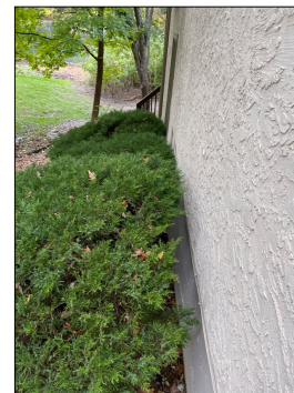
Prune or remove any plants that are in contact or within 12" of home to eliminate water damage to the siding surfaces or pathways for wood destroying insects.
