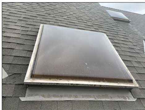
The Skylight(s) appear to beyond their life expectancy. Recommend replacement. MONITOR
