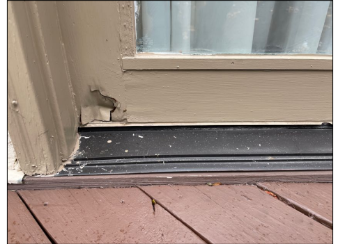
The north stationary section has wood damage. When I push on the surface it collapsed.
