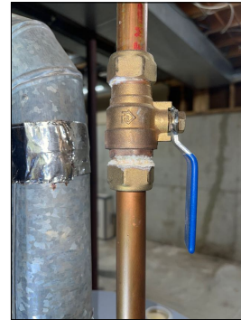
Evidence of a leak at the cold water shut off valve connection
