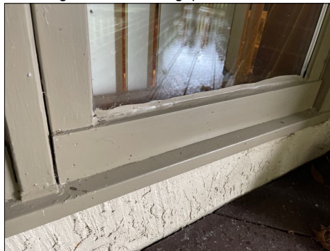
The triple casement windows on the lower deck north side of the brick chimney are in poor condition and has had woods/trim attached to the bottom of the windows.
