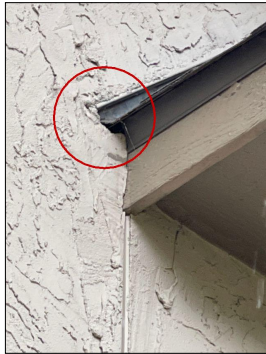
Missing Kick Out Flashing's need to be installed at: On the south side of the garage above the electric meter area.
