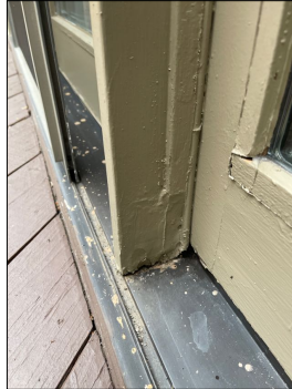
Water damage to the exterior vertical wood section between the opening door in the center stationary section.
