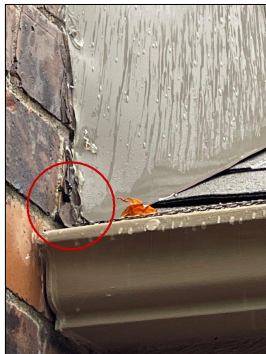
Missing roof kick out flashing on both sides of the chimney.
