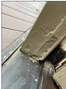
There is Water Damage at the Door Casement south side. The north side has been replaced
