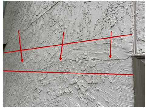
The south side of the Home Stucco surfaces has quite a few vertical cracks but also has a larger horizontal crack at the lower level west of the air conditioning condenser at a window. The smaller cracks can be skim coated but the horizontal crack appears to have loose material and may need to be removed and replaced.
