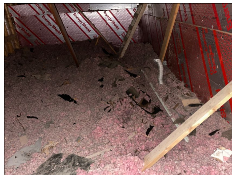
There has been foot traffic in areas in the attic which has lowered the height of the insulation that should be corrected.
