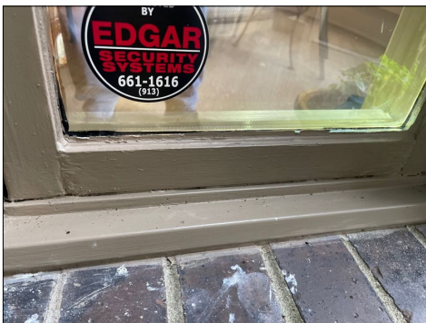
The kitchen breakfast nook bay windows, both of the south windows have rotted window extrusions and bottom window casement.
