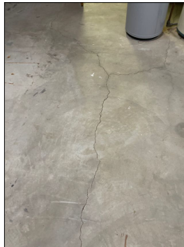
Typical slab cracking.
