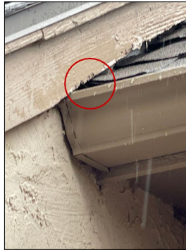
Missing roof kick out flashing on the west side at the north end of the gutter north of the chimney area.
