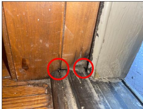
The casement has a gap at the weatherstrip that leads inside
