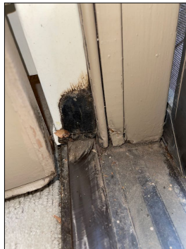
There is Water Damage at the Door Casement.
