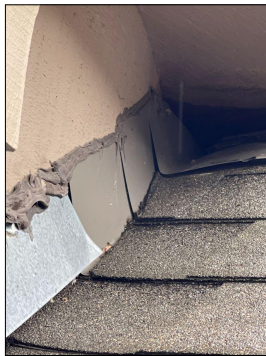
The kitchen area around brick structure on the north side does not have proper counter flashing at the top area in the lower galvanized counter. Flashing is not properly sealed and then the bottom step flashing above the eave does not have a kick out flashing and it is also not sealed properly. ** May need to fit trim to cover as well. **
