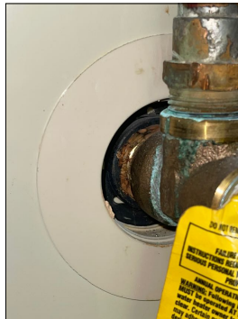
The TPR Valve is upside down!
