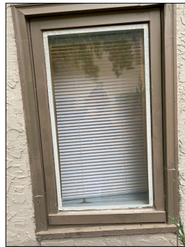
Southside lower window west of the air condition condenser is in very poor condition. Brick molding has been patched in with sections, the window sags and there is a gap at the bottom.
