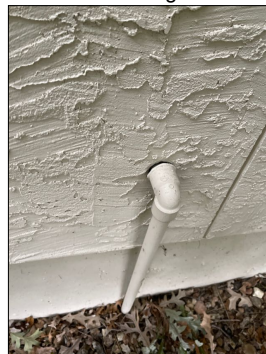
Need to seal up around the exterior sprinkler system electrical conduit on the south side of the garage.
