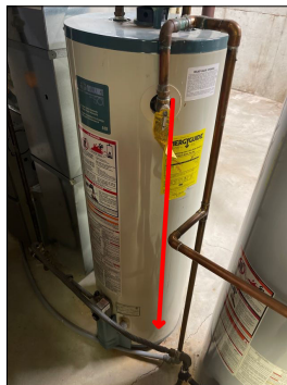
The TPR Valve Discharge piping installed is not allowed and need to install a properly approved Discharge pipe that stops 6" above the floor surface.
