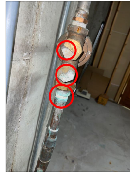
Evidence of corrosion at the pressure regulator and the pressure regulator connection
