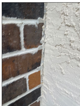
The brick chimney eyebrows need to be sealed with a brick meets the stucco and then down the vertical sides of the brick also needs to have new sealant applied.
