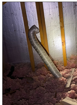
On the far south wall there is an exhaust hose that's pushed up against the exterior surfaces and needs to be redirected.
