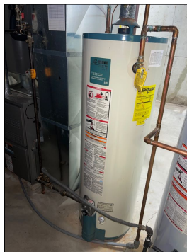
IPR Valve is upside down.
