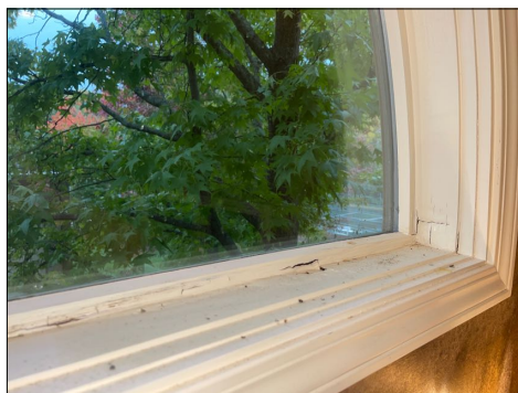
The picture window bottom interior casement and sill is rotted out
