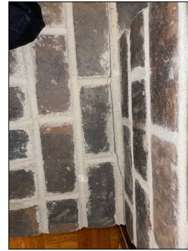
Hearth crack along the north end
