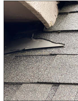
There is a shingle tab lying in the gutter above the kitchen roof area. It appears to have broken loose below the gutter area where there's flashing located.
