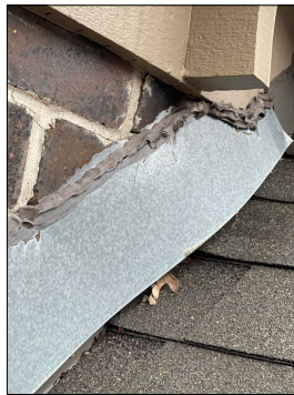
The kitchen area around brick structure on the north side does not have proper counter flashing at the top area in the lower galvanized counter. Flashing is not properly sealed and then the bottom step flashing above the eave does not have a kick out flashing and it is also not sealed properly.
