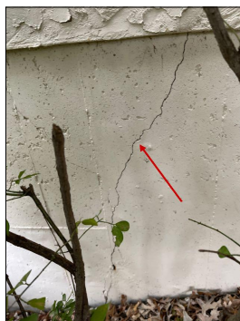
The southside foundation at the garage area has a couple of cracks which appear to be having some movement. The drainage is extremely bad along the side which causes issues with the foundation.
