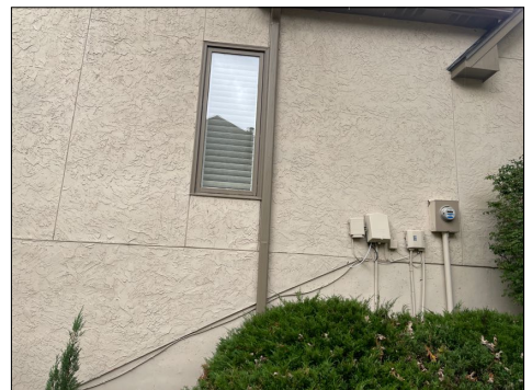
The casement window on the southside between the electric meter and the air conditioning condenser has water damage to the window glass extrusions in the bottom casement and sill area.
