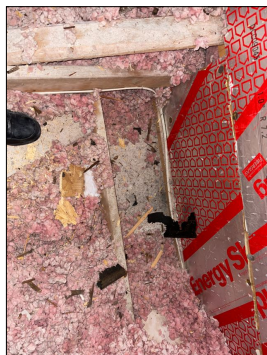
Visible ceiling drywall in a few areas where the ceiling joist are not covered with insulation. Need additional insulation. West of the garage area
