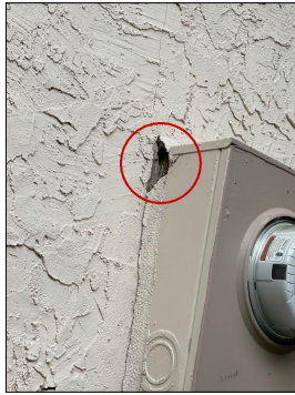
Water is getting in behind the main electric meter at the stucco surfaces causing water damage behind the stucco surfaces at the electric meter and the cable boxes. This area will need to be cut out and repaired.
