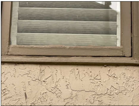
The casement window on the southside between the electric meter and the air conditioning condenser has water damage to the window glass extrusions in the bottom casement and sill area.
