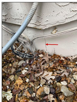
Foundation crack noted behind the air conditioning condenser.
