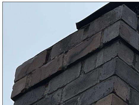
The chimney top concrete crown should be skim coated in the top two rows of brick need some minor tuck pointing.
