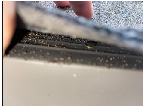
The eave Metal drip edges are installed on top of the felt paper/underlayment material instead of under the felt paper/underlayment material per manufacturers installation guidelines. This is also required by the majority of the City Codes.
