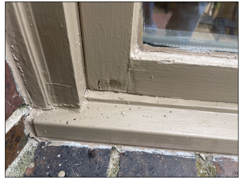
The kitchen breakfast nook bay windows, both of the south windows have rotted window glass rails and sash and bottom window casement.
