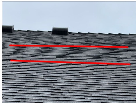
On the west side of the roof towards the southside center area is a raised/Humped Area of the roof surface. It is approximately 6 feet in length and approximately 2 feet high. This needs to be evaluated and corrected.
