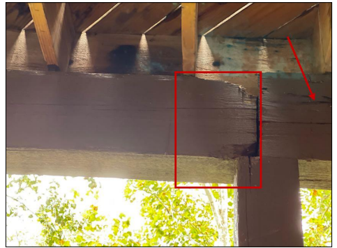
The upper deck west side Girder/Support Beam has water damage and also evidence of carpenter bees. Due to the height and size of the structure I am recommending further evaluation and possible replacement.
