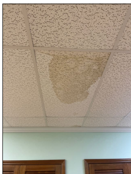
Evidence of Water Stains noted at: center of room
