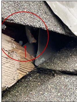
The kitchen round brick structure northside at the bottom of the valley there are openings above the flashing and also some wood damage that doesn't help. This needs to be properly flashed now.
