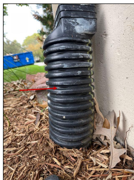
The downspout underground drain pipes are perforated/slotted and CAN'T be used for downspouts.
