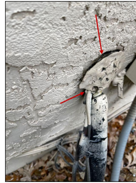
Need to seal up around the exterior air-conditioning refrigerant lines were enters the siding with Thumb Gum Sealant.
