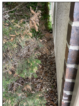
POOR DRAINAGE-CORRECT NOW, Southside all
