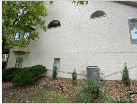
The south side of the Home Stucco surfaces has quite a few vertical cracks but also has a larger horizontal crack at the lower level west of the air conditioning condenser at a window. The smaller cracks can be skim coated Betty horizontal crack appears to have loose material and may need to be removed and replaced.
