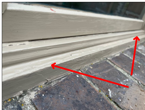
Garage north side windows has water damage to the bottom casement sill area at the brick.
