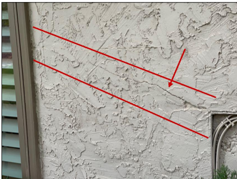
The south side of the Home Stucco surfaces has quite a few vertical cracks but also has a larger horizontal crack at the lower level west of the air conditioning condenser at a window. The smaller cracks can be skim coated Betty horizontal crack appears to have loose material and may need to be removed and replaced.
