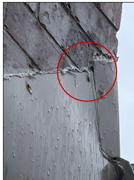
The metal roof flashing of course is attached to the surface of the chimney brick and the sealant along the top of the counter flashing will need to be checked every three years. ** There are areas now that need to be sealed **
