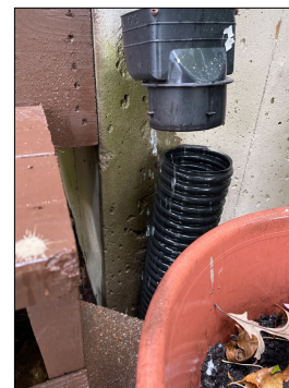
The far south west corner downspout has become disconnected from the underground drain pipe and is dumping water against the foundation. There should be a reducer that extends down into the underground pipe at least 8 inches to prevent this. The downspout should never be securely attached to the underground pipe.
