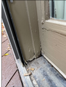
The exterior vertical divider between the main door in the station in the door has water damage.
