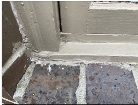
Kitchen breakfast nook bay window second window from the north side has water damage to the bottom of window casement and the window sill.
