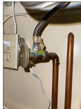
Evidence of a leak at the hot water shut off valve
