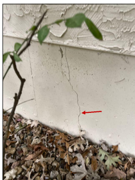
The southside foundation at the garage area has a couple of cracks which appear to be having some movement. The drainage is extremely bad along the side which causes issues with the foundation.
