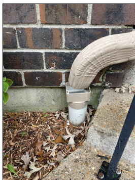
The downspout at the front porch is supposed to be emptying into an underground drain and it needs a reducer installed on the downspout so it goes down inside the underground pipe.
