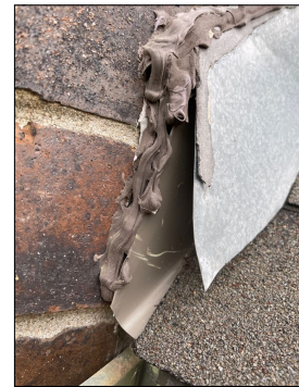
The kitchen area around brick structure on the north side does not have proper counter flashing at the top area in the lower galvanized counter. Flashing is not properly sealed and then the bottom step flashing above the eave does not have a kick out flashing and it is also not sealed properly.
