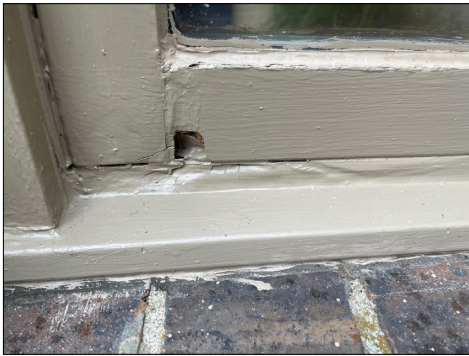
The kitchen breakfast nook bay window, north window bottom frame and window glass rails and sash are rotted out.
