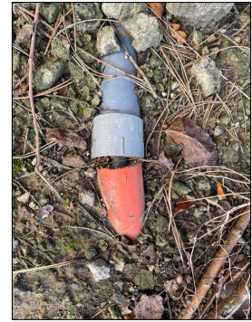
On the exterior Northside north west corner there is an electrical conduit next to the building surface and the conduit has separated leaving the cable exposed.
