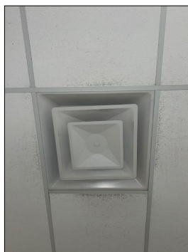
Evidence of Mold-Like substance and further evaluation is recommended. Located: Surrounding west hall supply vent
