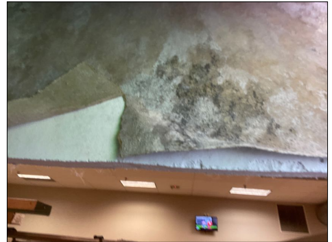
Orange room west wall mold growth above wall cut out at the higher wall cut out areas.
