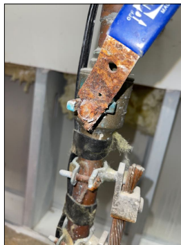
Shut off valve is very rusted. Recommend replacing
