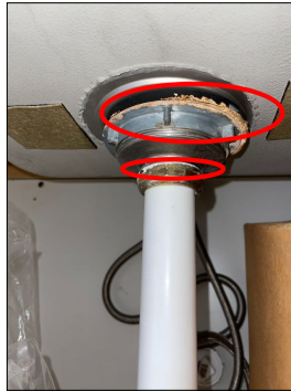
Evidence of a leak at the sink flange and the drain connection
