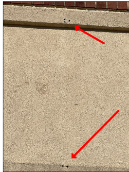
There are areas of the front drivit stucco material That has holes to the surfaces that needs to be repaired. Check all incorrect as needed.
