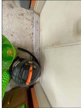
There is Water Damage at the Door Casement and door itself
