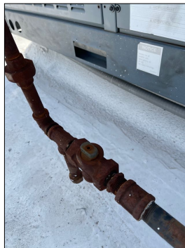
Gas Valve Present
