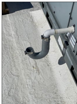
The air conditioning condensation drain needs to be extended to the west roof drain.
