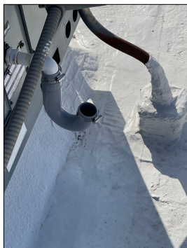
Air conditioning condensation drain line needs to be extended to the west roof drain.
