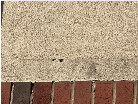
There are areas of the front drivit stucco material That has holes to the surfaces that needs to be repaired. Check all incorrect as needed.
