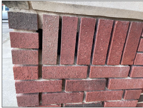
There are several areas of the exterior brick where the mortar is deteriorated and needs to be cleaned up and tuck pointed.
