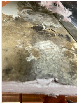
Orange wall mold growth found Above wall cut out where the electric panel is located and the kennel to the north of it.
