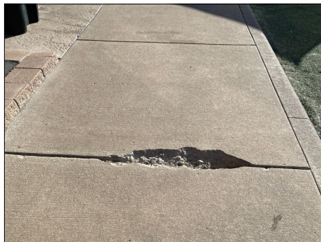
Southside sidewalk at Pet exterior play area is a large opening and is a tripping hazard.
