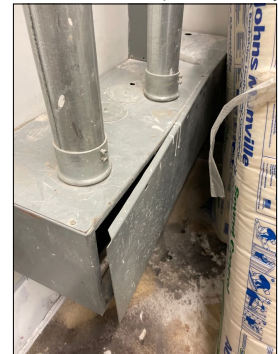
In the west electric panel room where the main water shut off valve is located, just to the north side is an electrical race and the cover is loose leaving the interior wiring exposed and Unsafe. There are also missing knockout plugs that needs to have plugs installed.
