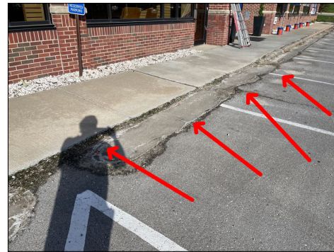
The sidewalk handicap ramp area is completely deteriorated.
