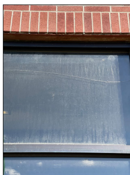
Window Pane Glass is Cracked/Broken at: Center exterior doors above it to the east top window.
