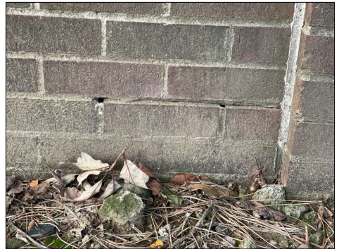
There are several areas of the exterior brick where the mortar is deteriorated and needs to be cleaned up and tuck pointed.
