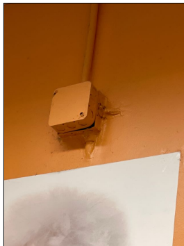
Junction box not sitting flush with second box at: north boarding sw corner west wall
