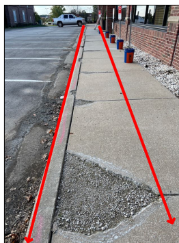
Sidewalk deterioration along the front sidewalk area.
