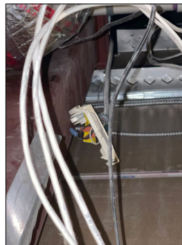
Junction Boxes missing either Cable Connectors, Cover or Knock-Out Plugs at: above west side sw corner room
