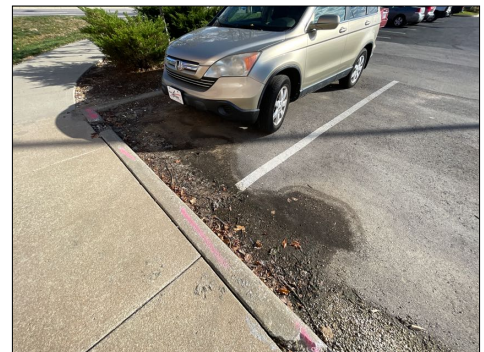
Water is sitting along the front of the building at the concrete curb area due to the parking lot sloping towards the curb.
