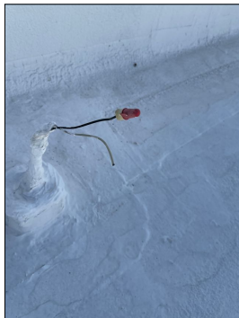
There is open electrical on the roof along the east side south of center. These are not properly capped off either in a junction box or they need to be disconnected from the electrical system.
