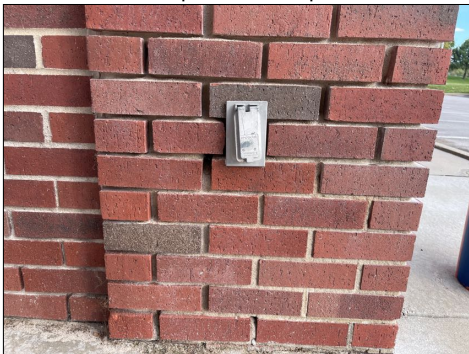
There are several areas of the exterior brick where the mortar is deteriorated and needs to be cleaned up and tuck pointed.
