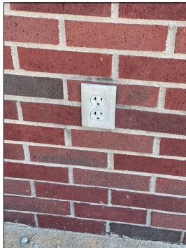
Exterior west side at the center of the building is an electrical receptacle that is dead plus it does not have an exterior cover installed.
