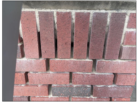
There are several areas of the exterior brick where the mortar is deteriorated and needs to be cleaned up and tuck pointed.
