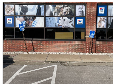
The Handicap signs are missing or damaged. Corrections required. Both signs need to be reset. They are very loose and ready to fall over.
