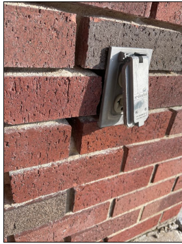
The Exterior Receptacle Cover is Damaged at: Front entrance,
