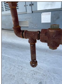
Sediment Drip Leg Present
