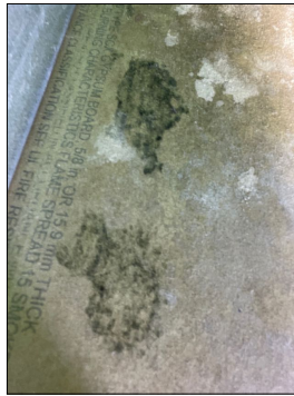
Orange room west wall mold growth above wall cut out at the higher wall cut out areas.
