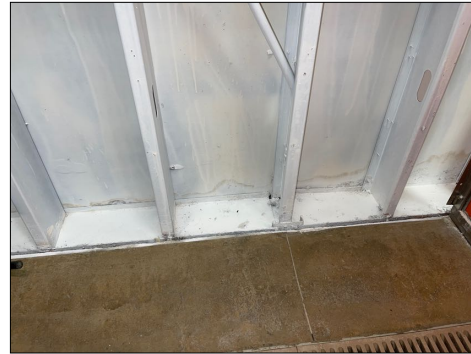
Evidence of a Mold-Like substance present. Mold Testing or Mold Remediation may be required. RC Certified Inspections can provide these services. Also see the MOLD Growth Section in the report. This was found at: found in north boarding room west white walls along floor
