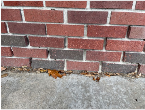
There are several areas of the exterior brick where the mortar is deteriorated and needs to be cleaned up and tuck pointed.
