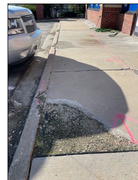
Sidewalk deterioration along the front sidewalk area.
