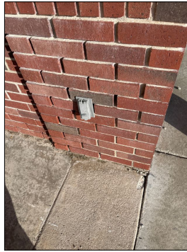
The receptacle at the front entry was dead at the time of the inspection. There may be a GFCI receptacle on the interior.
