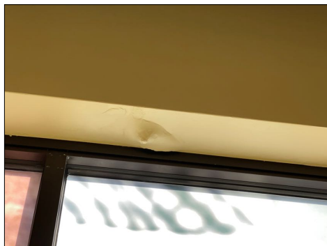
Damaged wall due to water intrusion: North side above the east wall south set of windows
