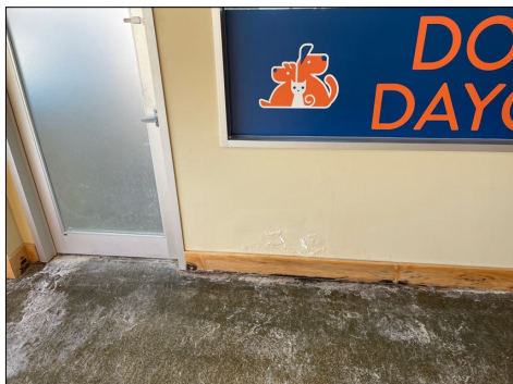
Evidence of a Mold-Like substance present. Mold Testing or Mold Remediation may be required. RC Certified Inspections can provide these services. Also see the MOLD Growth Section in the report. This was found at: along south wall - presumably due to dog pee
