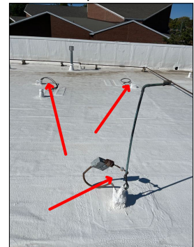
There are three unused old HVAC electrical systems at the center west side area. The lines appear to be dead. Recommend verification and disconnect and clean up of these systems.
