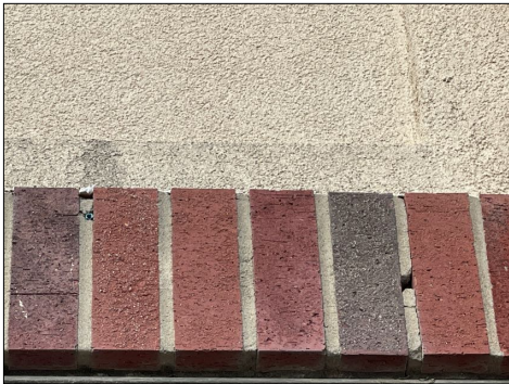
There are several areas of the exterior brick where the mortar is deteriorated and needs to be cleaned up and tuck pointed.
