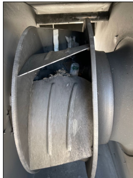
There is debris in the rotating fan blades.
