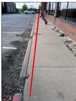
Tripping hazard(s) noted:
