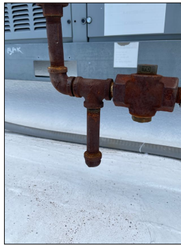
Sediment Drip Leg Present
