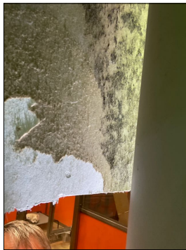
Orange room west wall mold growth above wall cut out at the higher wall cut out areas.
