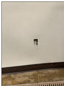
Missing or Damaged Receptacle Covers at: west boarding east wall 2nd dog pin from north
