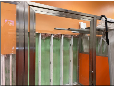
Orange room west wall mold growth above wall cut out at the higher wall cut out areas.
