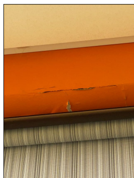
There is evidence of moisture intrusion noted. We are recommending water intrusion investigation. Water intrusion could develop mold growth on the surfaces. RC Certified Inspections can provide this investigation. Located at: East Exam room above windows
