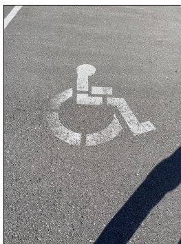
It is recommended that the handicap parking lot striping to be re-striped. They are faded and should be corrected.
