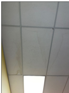
Evidence of Water Stains noted at: above the east door (could be caused by old roof)
