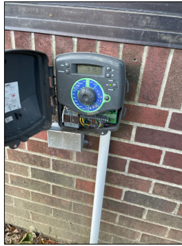
The sprinkler system control panel is located On the exterior northside north west corner.
