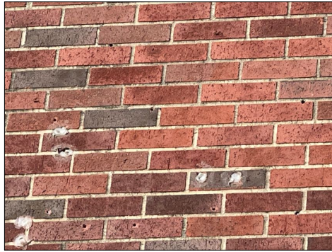
There are areas on the front of building at the upper brick where it looks like there has been signs installed and there are holes in the surface of the brick and mortar that should be sealed or tuck pointed.
