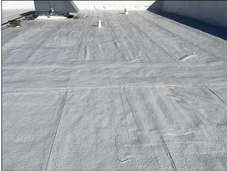
There are a lot of bubbles and wrinkles in this old rolled asphalt material. There are also several areas that it been patched.
