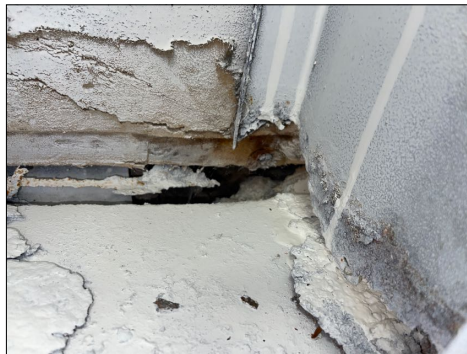
Void under the center west wall in the north boarding room
