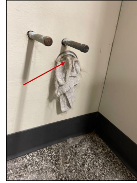
Grooming room east wall north end has a drain pipe that was not capped off properly.
