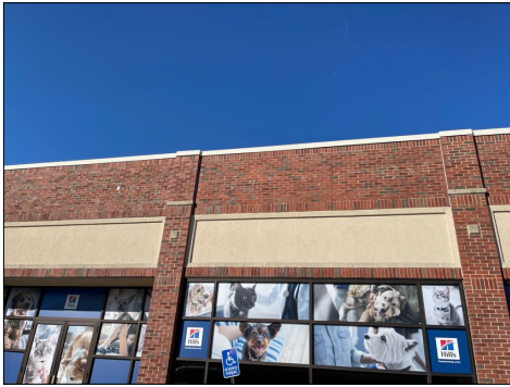
There are areas on the front of building at the upper brick where it looks like there has been signs installed and there are holes in the surface of the brick and mortar that should be sealed or tuck pointed.
