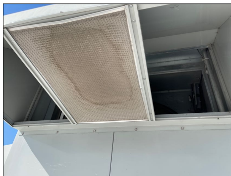
There are three prefilters on the exterior and two of them are missing and the one present is very dirty.
