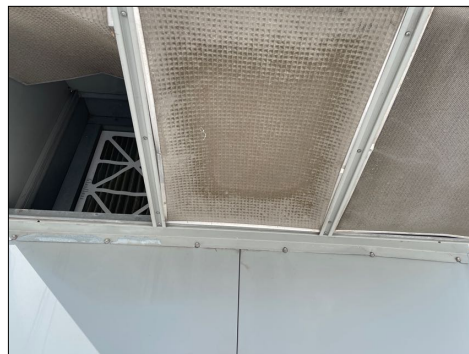
One of the prefilters are missing.
