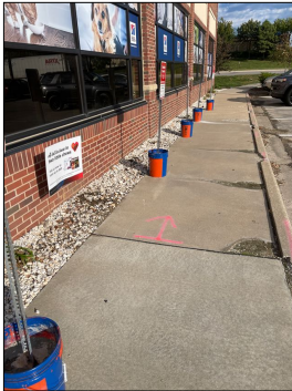
Along the front east side of the building between the brick foundation and sidewalk area is soil with no evidence of drainage. This is keeping water trapped between the sidewalk and the brick surfaces.
