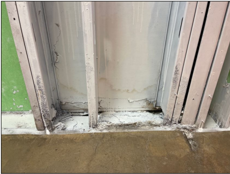
west wall in the north boarding room has water staining at the floor along the white painted walls
