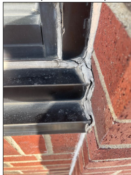
Exterior store front windows and bottom sill trim areas have sealant that is missing or opened. Need to clean up these areas and reseal.
