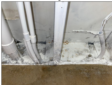
Void under the west wall in the north boarding room under electric panel
