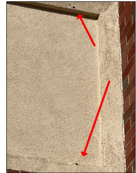
There are areas of the front drivit stucco material That has holes to the surfaces that needs to be repaired. Check all incorrect as needed.
