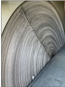
The circular rotating fins are badly damaged because of air filters being loose and laying up against the surfaces on both sides. Complete evaluation required.
