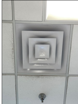
Evidence of Mold-Like substance and further evaluation is recommended.
