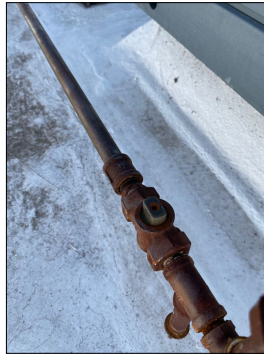
Gas Valve Present
