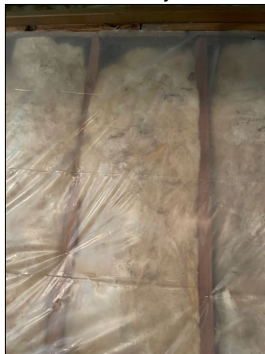
There is mold growth between the exterior wall insulation and vapor barrier in the basement due to elevated humidity.
