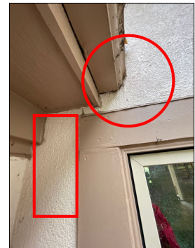
On the exterior west side of the living room above the north side windows there is a gutter there is excessive moisture content at the gutter area and below the soffit proximately 12 inches.
