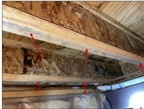
Mold growth along the bottom of several floor joists in the basement
