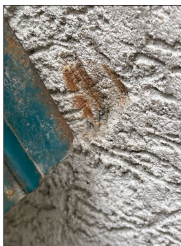
Need to remove the southside garden hose bracket that is attached to the siding. Should not have this attached to the synthetic stucco surfaces and the bracket has also dug into the surfaces.
