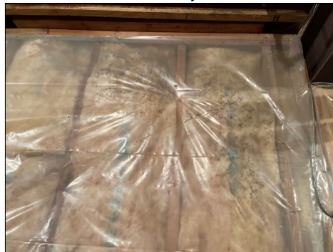
There is mold growth between the exterior wall insulation and vapor barrier in the basement due to elevated humidity.
