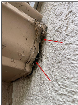
The synthetic stucco mesh is visible at the end of the gutter above the living room exterior above the North side of the window. This may be where the moisture is getting in behind the surfaces.
