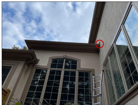
Living room area. West side above the living room south side windows at the gutter running north to south, the kick out flashing was not installed properly and there is visible EIFS Base Coat Mesh at the end of the guttering.
