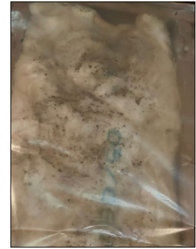
There is mold growth between the exterior wall insulation and vapor barrier in the basement due to elevated humidity.
