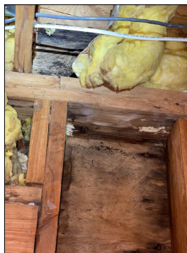
Mold growth is visible in the basement on the exterior wall sheathing at the southside of the exterior pedestrian doors. This is from water intrusion from above the northside living room windows area.
