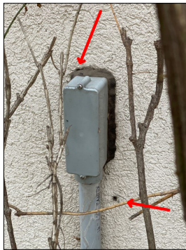
On the west side south of the air conditioning condensers, there's electrical conduit that needs to be sealed up and there's also screw hole that needs to be sealed.
