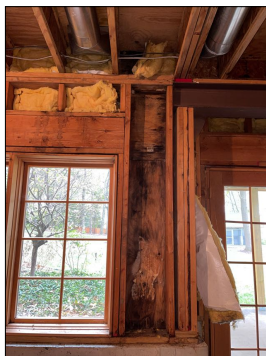
Mold growth is visible in the basement on the exterior wall sheathing at the southside of the exterior pedestrian doors. This is from water intrusion from above the northside living room windows area.
