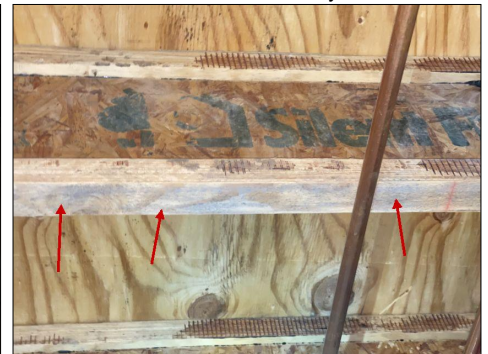
Mold growth along the bottom of several floor joists in the basement
